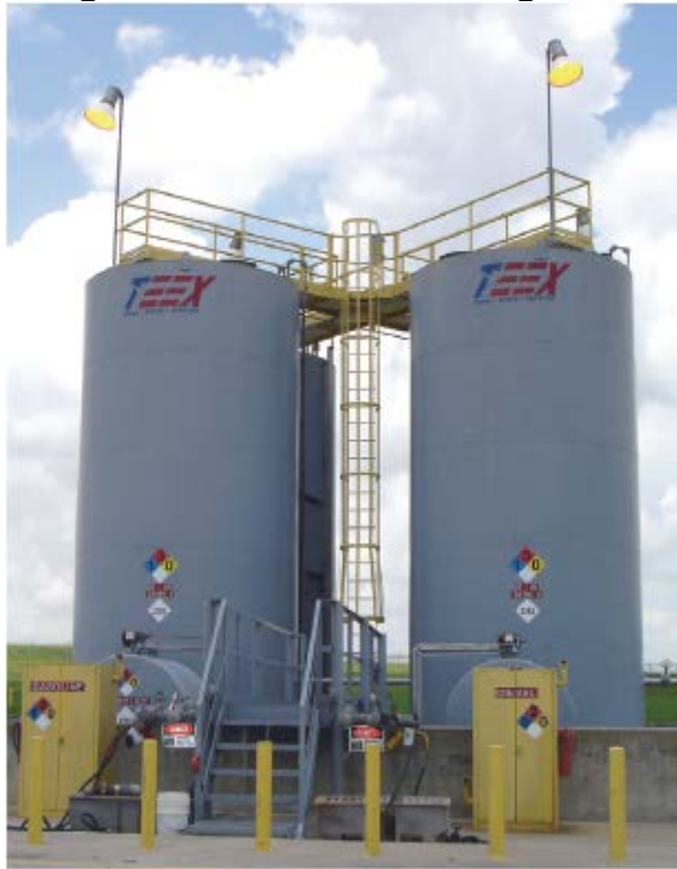
Figure 4.1: Cone Roof Storage Tank
