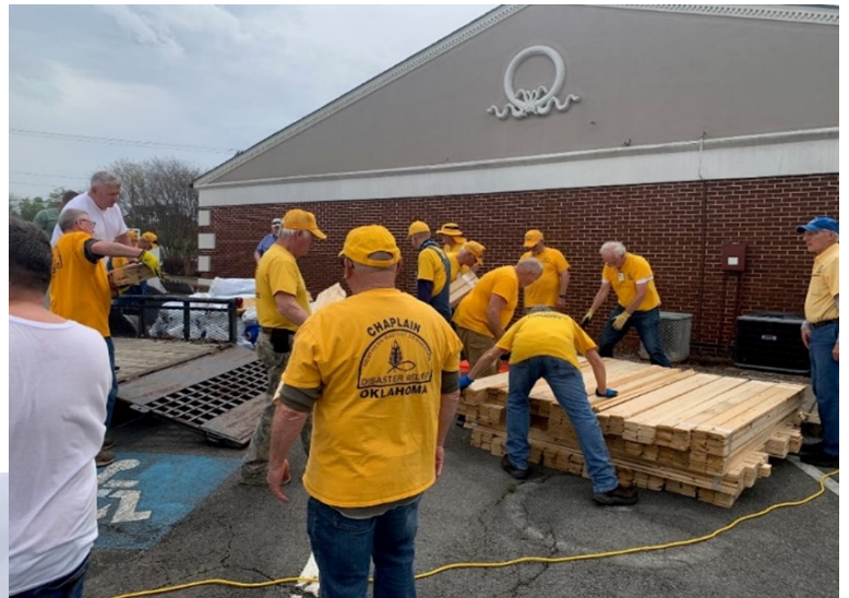
Right: Baptist Disaster Relief team working with ADEM staff to off-load tarps and wood slats for installing the tarps. These resources were provided through ADEM and made available to jurisdictions, as requested, to cover damaged homes.
