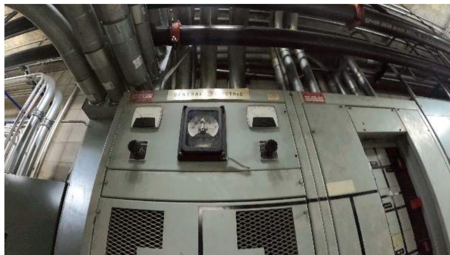
Image: Metering the original service equipment.
