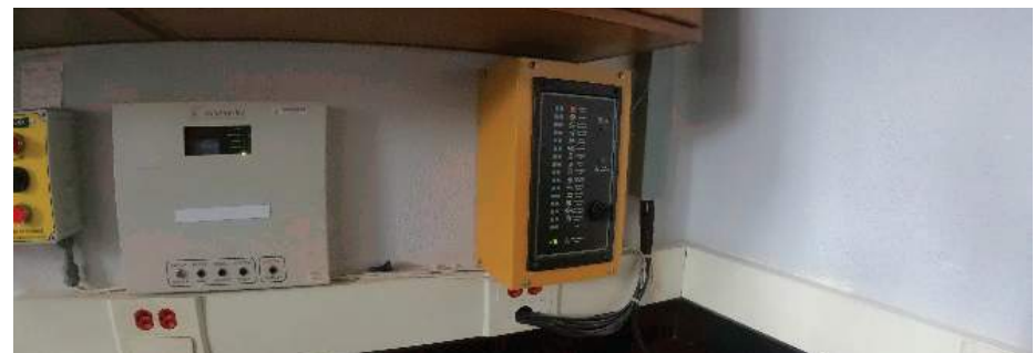
Image: Current generator monitoring panel.
