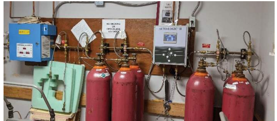
Image: Manifolded helium system. The medical air system (blue box) in the image is intended to be connected to local cylinders and is currently disconnected.
