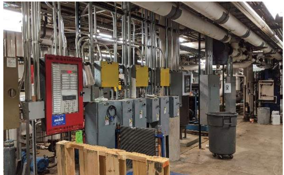
Images: FACP in Mechanical Room.
