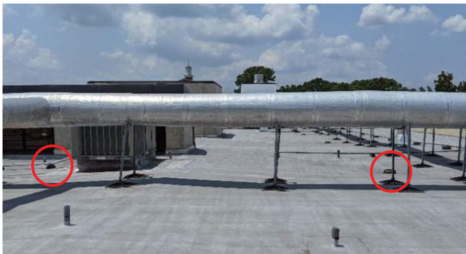
Image: Regular spacing of primary only roof drainage system (red circles) with no overflow drains or scuppers.
