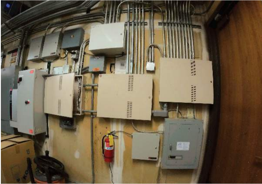
Image: Security equipment in the mechanical room.
