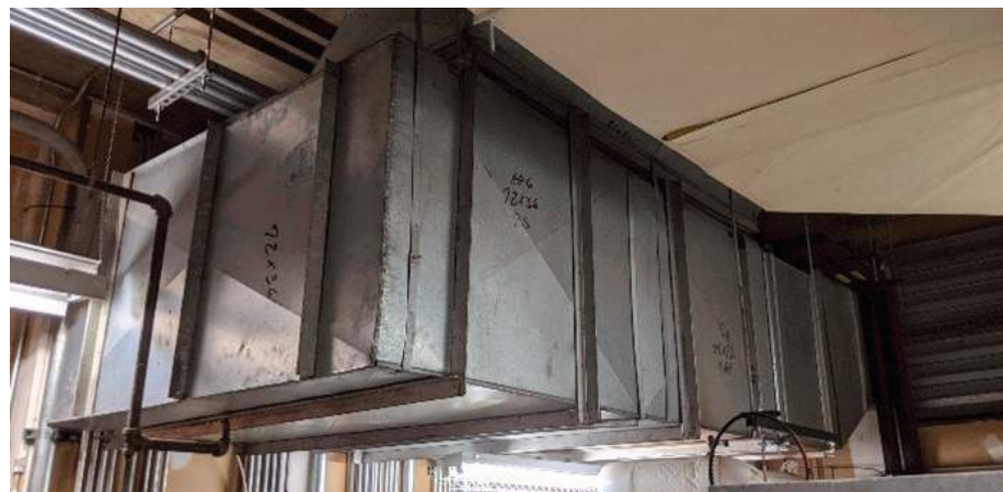
Images: Third-floor air-handling unit (1998) with tempered outside air chase from dedicated outside air heat recovery units.
