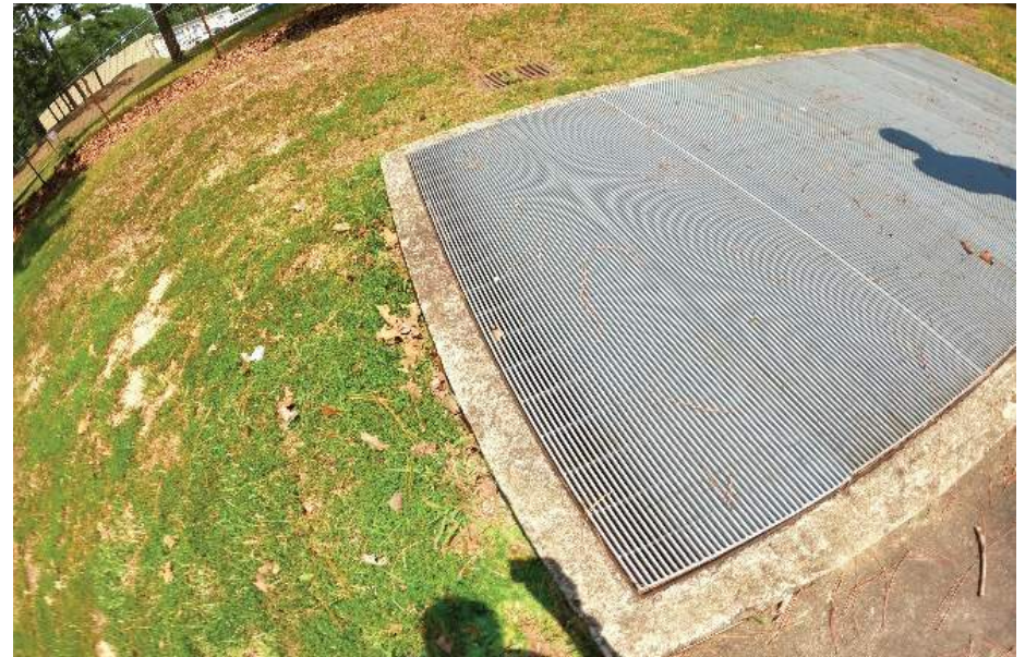
Image: Site Utility Vault Cover
