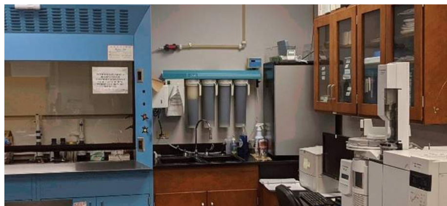
Images: Domestic cold-water entry in the basement central plant and a typical lab sink with gooseneck faucet but no vacuum breaker to protect domestic water source.
